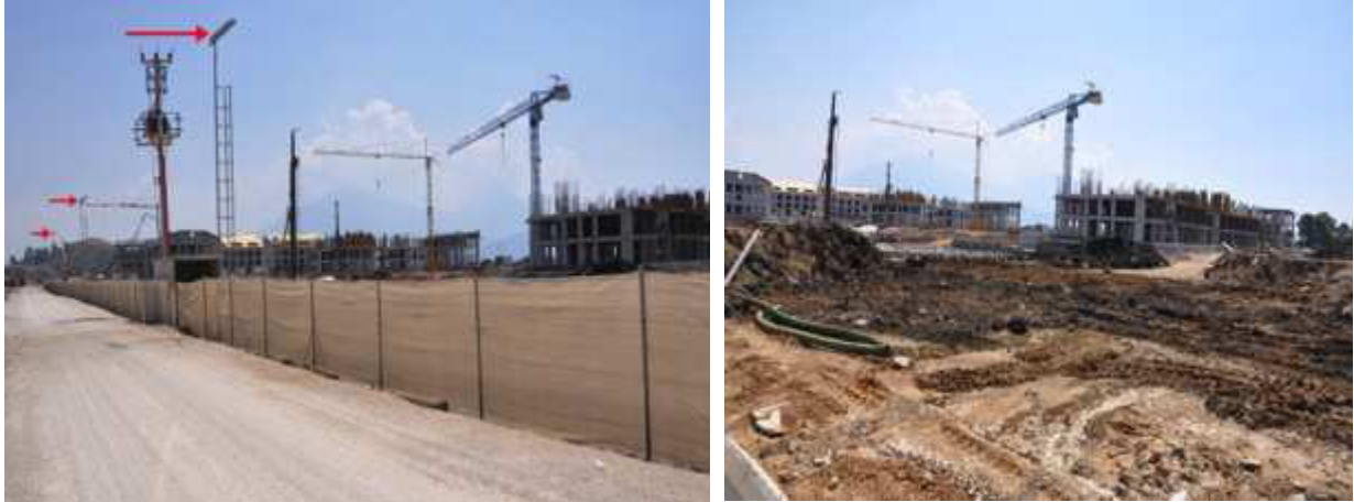
Fig. 59: Construction site Barut Hotel Fethiye (Photo: M. Stachowitsch), arrows mark the huge spotlights along the fence
