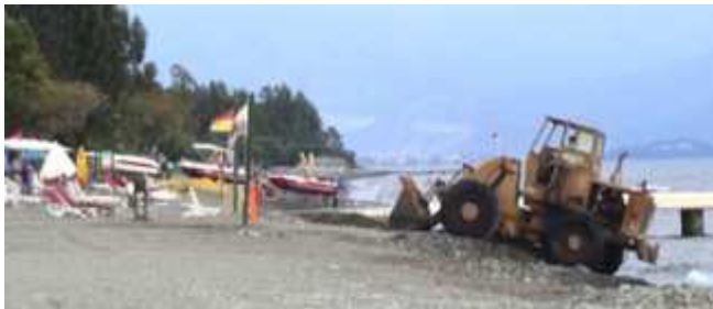
Fig. 38: Excavator restructuring the beach in front of Majestic Club Tuana (Photo: M. Herzog)
